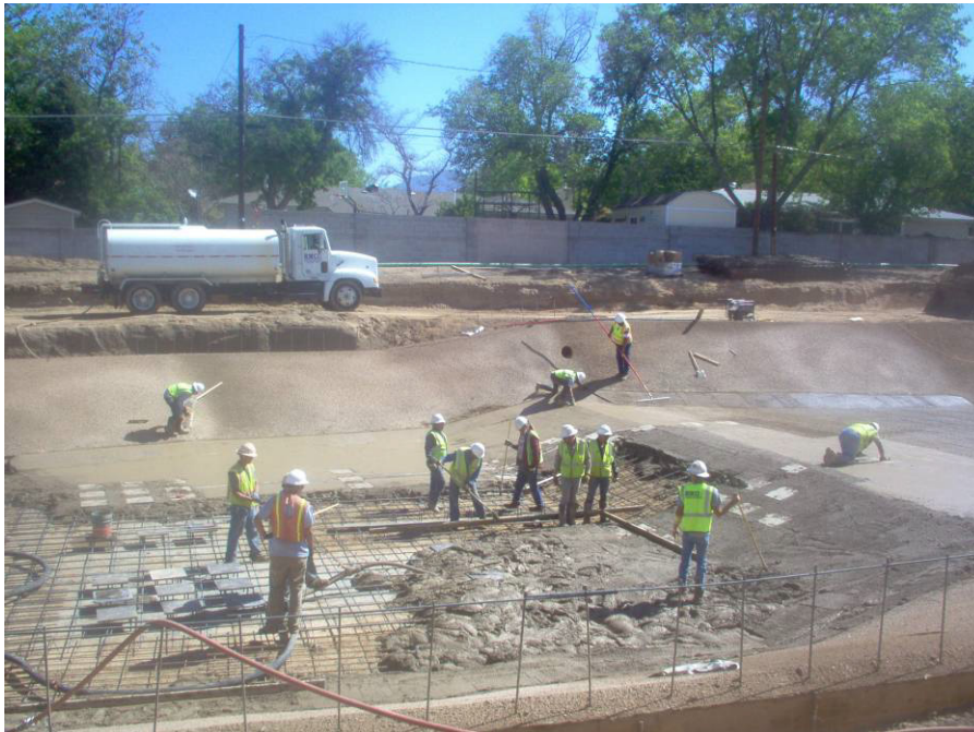
Superior pumping the shotcrete out with a 2 1/2" hose. RMCI crews finishing shotcrete.
