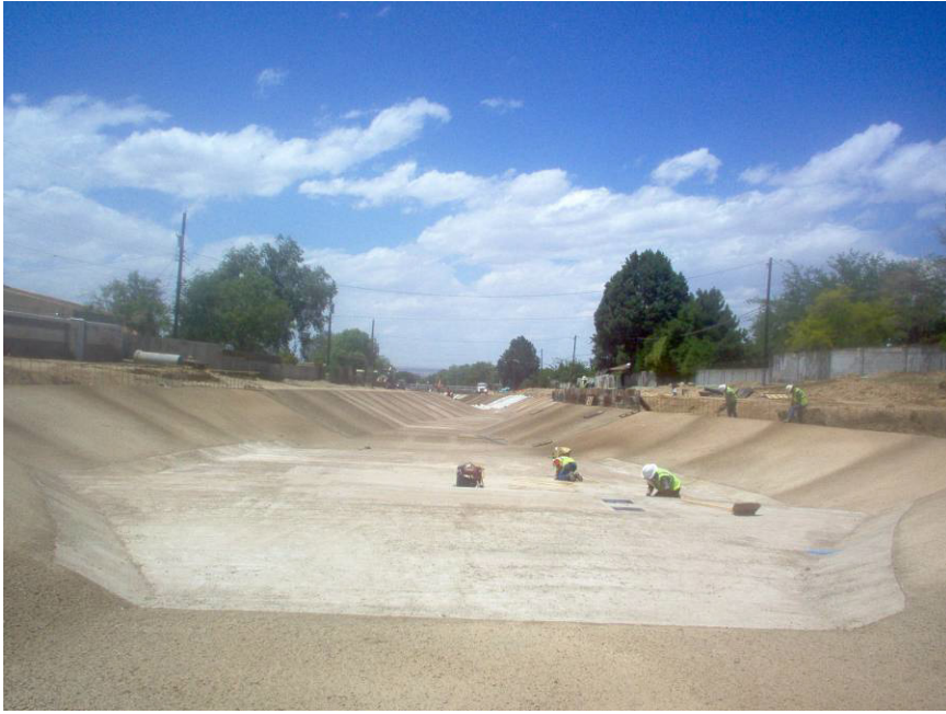
RMCI crews Cleaning the plates at the WQS and forming sill wall in the background.
