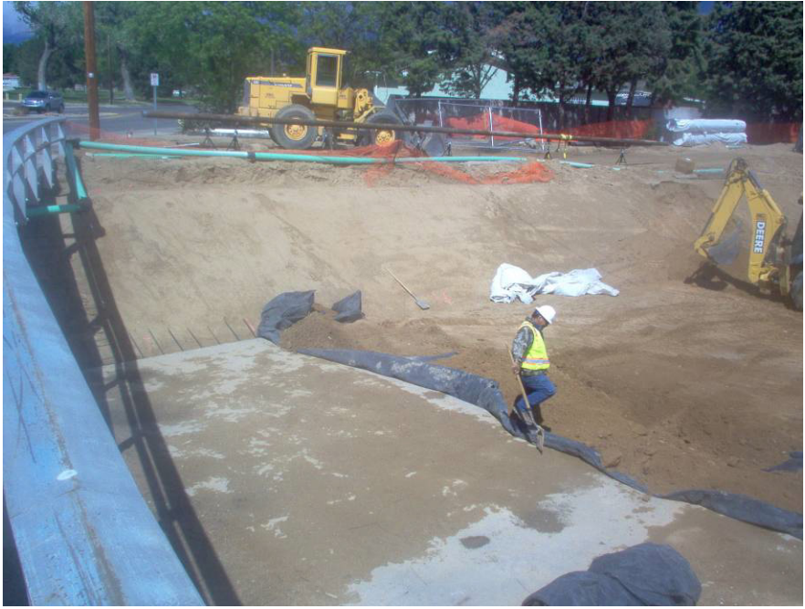
RMCI crew protecting the edge of the existing channel as storm drain waters threaten to wash down.
