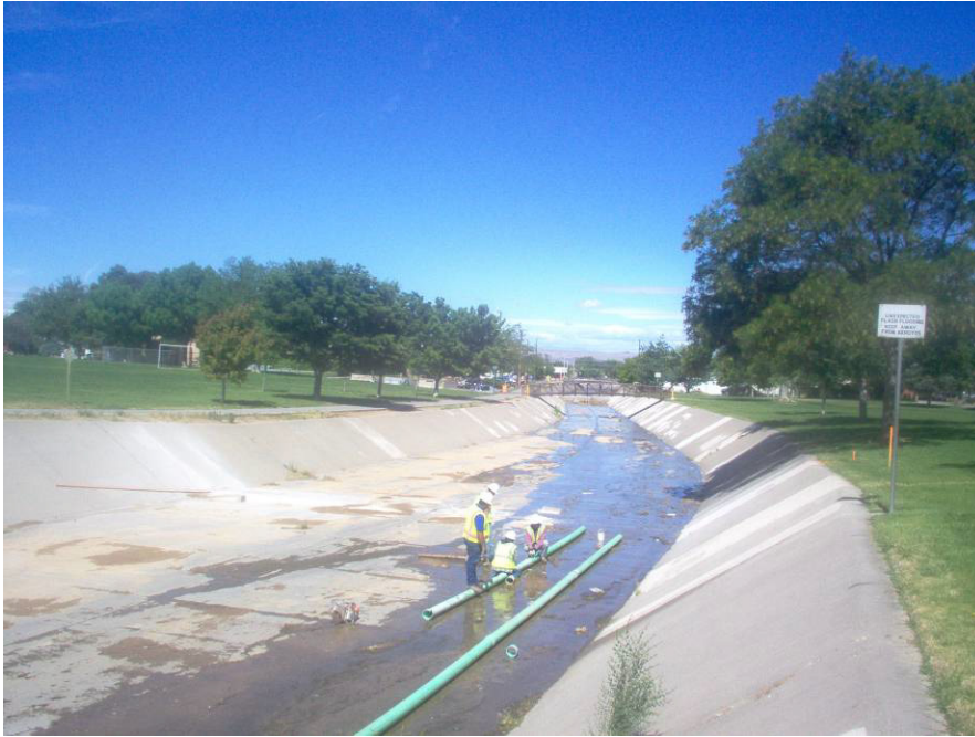
Crews extending the gravity drainline pipe to enable the contractor to cut channel for irrigation crossing.
