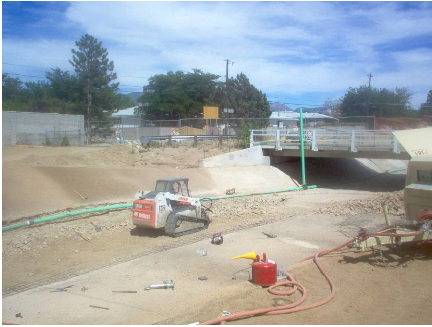
RMCI removing a portion of channel lining. Contractor worked late to finish removals.
