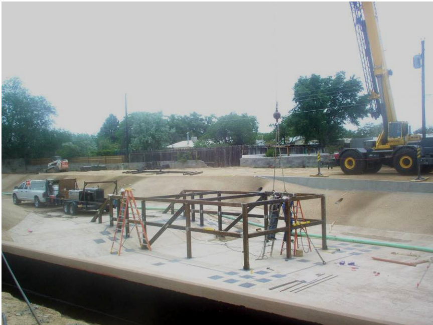
D&R Tank tack welded WQS in place. (Damp proofing on the back side of the sill wall.)
