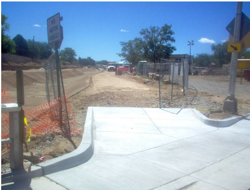
Bike Ramp/ Drive Pad on the SE corner of the San Pedro Bridge.
