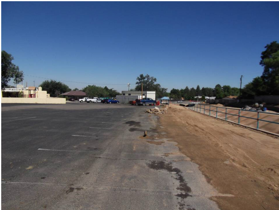
Main irrigation line has been placed here. There is some of the debris pulled from the trench.
