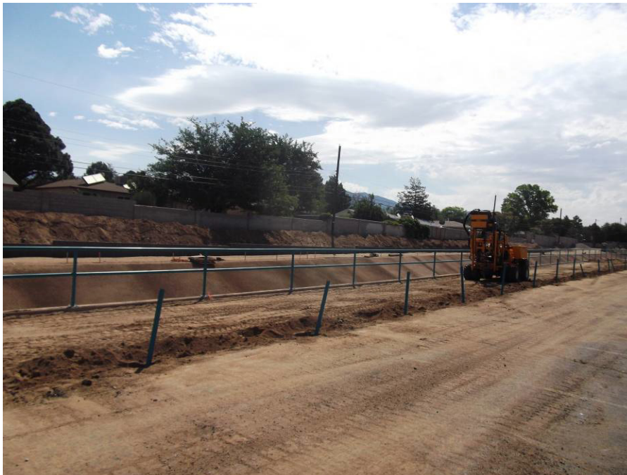
Scotts fence has drilled holes and began placing verticals with concrete in the pm
