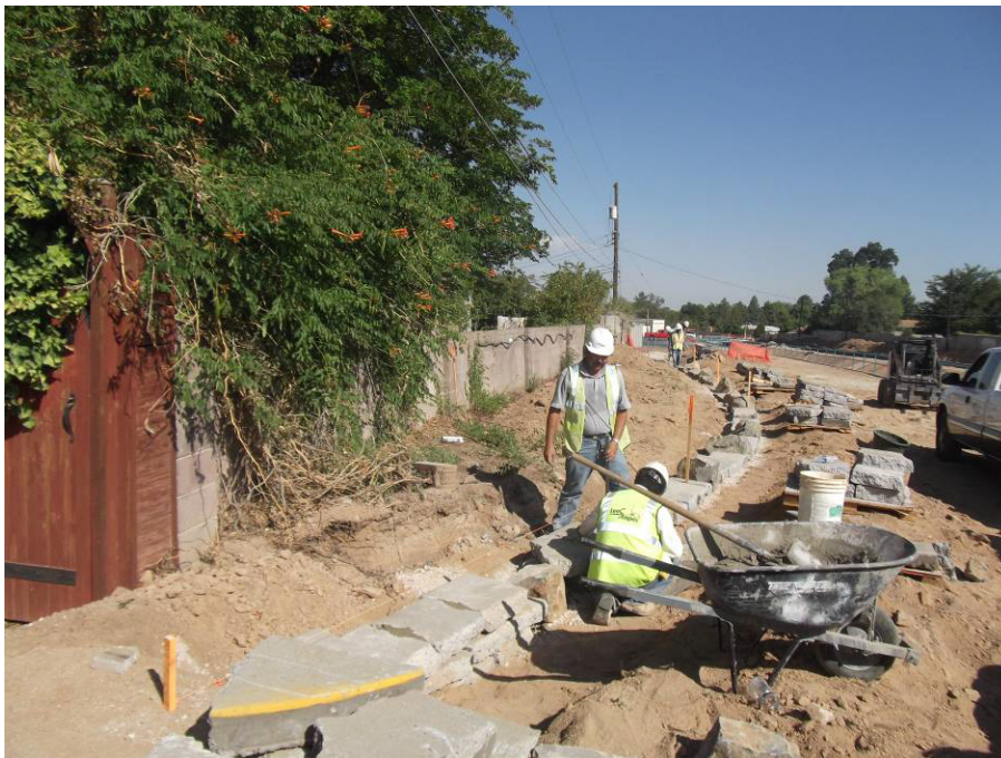
Leescapes working on seat wall west of California and south of the Channel
