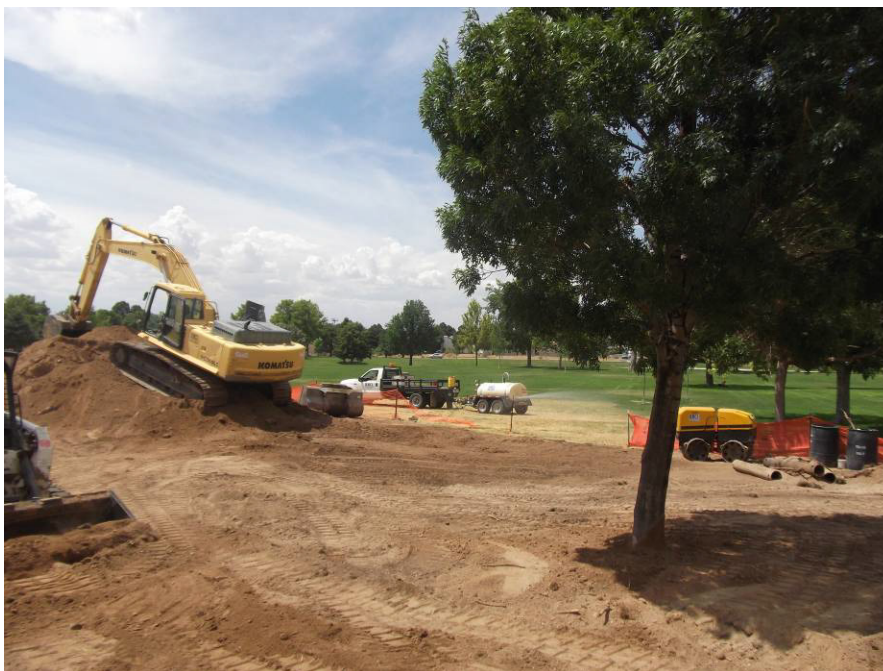
RMCI backfilling at Water Harvesting pipes and MH. Watering grass in the back ground.
