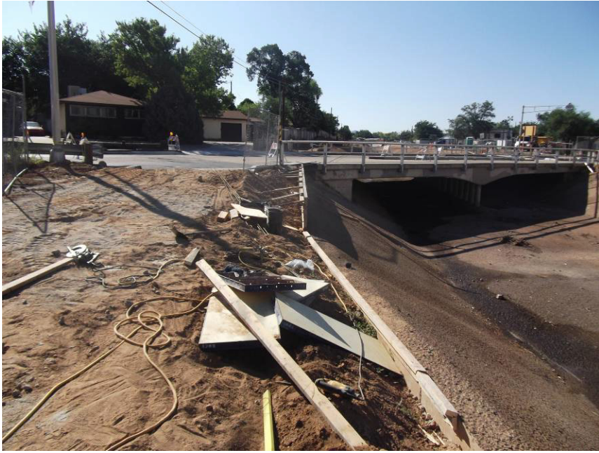
RMCI forming sill walls, this picture at the NW quad of the bridge and the channel
