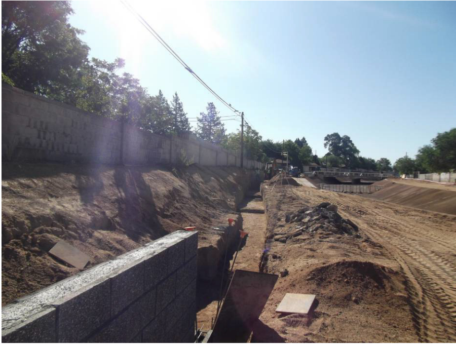
Peerless continues digging the footing on "B" wall – West of San Pedro North side of the channel
