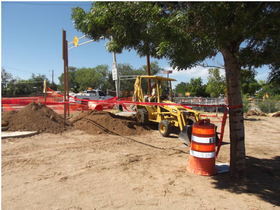
BEI – Bixby on site running power and placing controller
