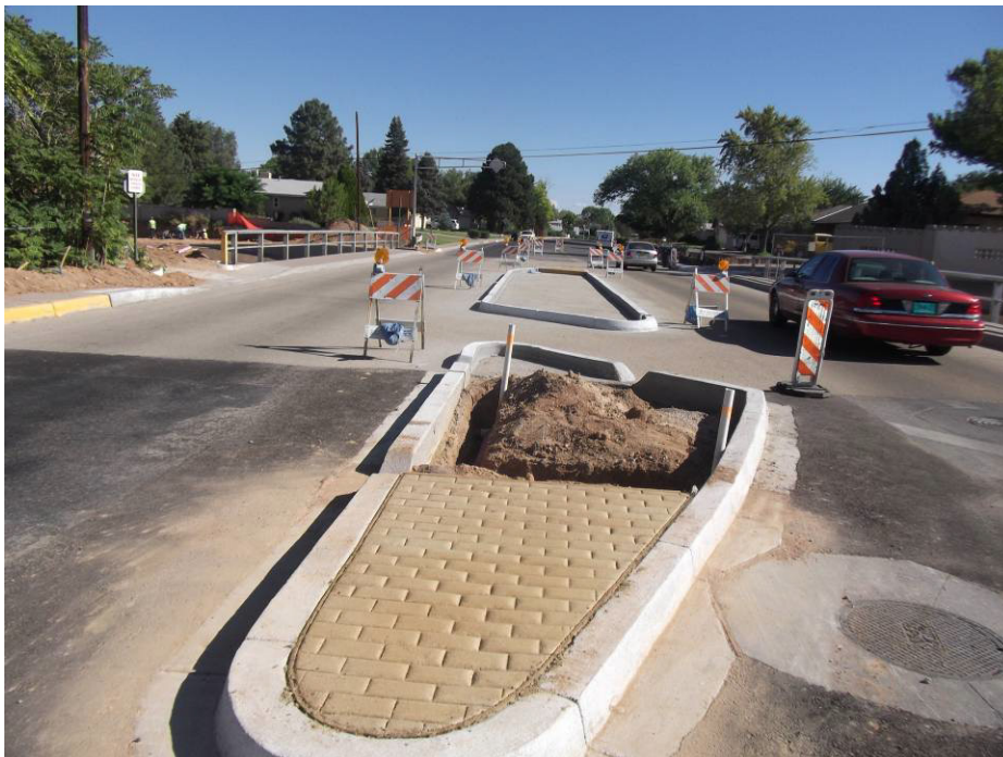
Median Noses placed yesterday by HO and Land Tek tying main line together at sleeves.
