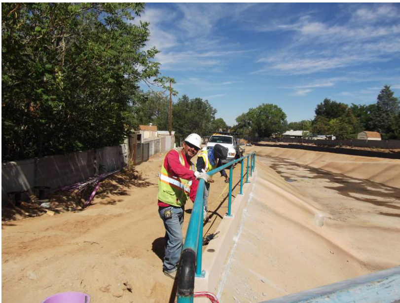
Scotts Fence working in the SW quad of the San Pedro Bridge placing pipe fence on Sill Wall.
