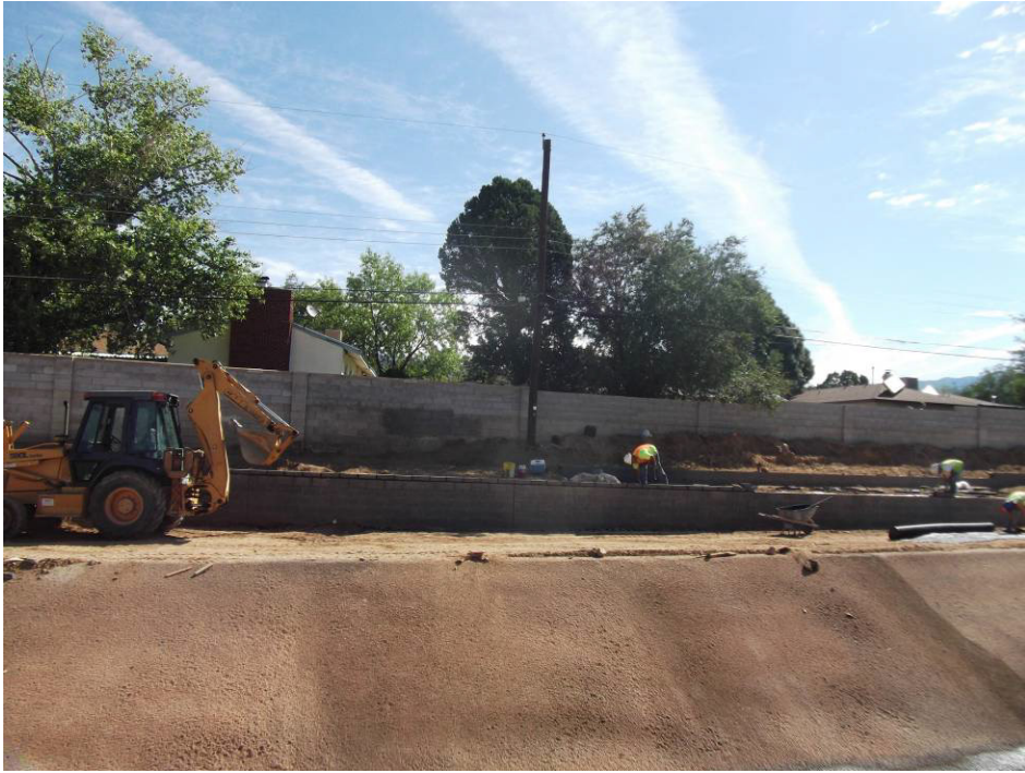
Peerless placing cap block on Wall "D" and clean up on Wall "C"
