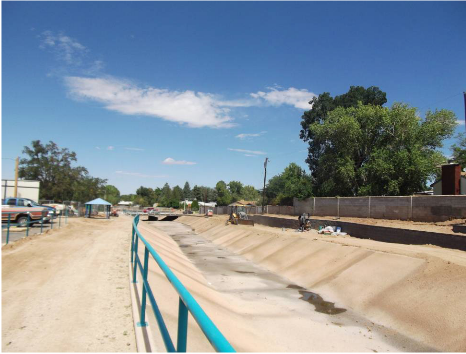
RMCI grading on the north side of the channel and digging out to place base course fillet.
