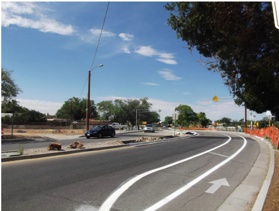
Land Tek placing 4-6" San Lazarus Cobble in the medians. COA crews painting stripes on Comanche.
