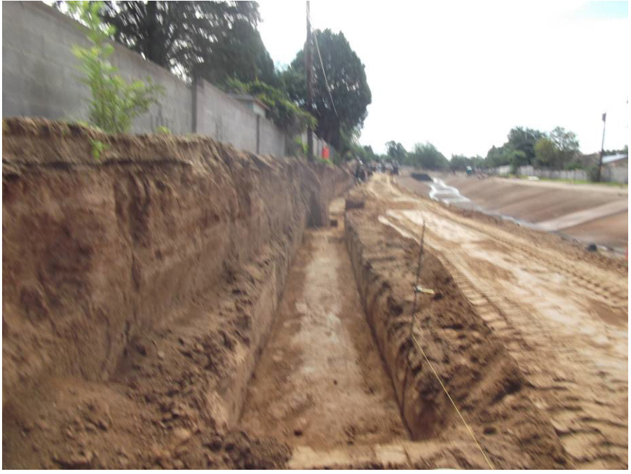
Footing for wall "A" – Contractor prepared "L" footing adjacent to utility pole.
