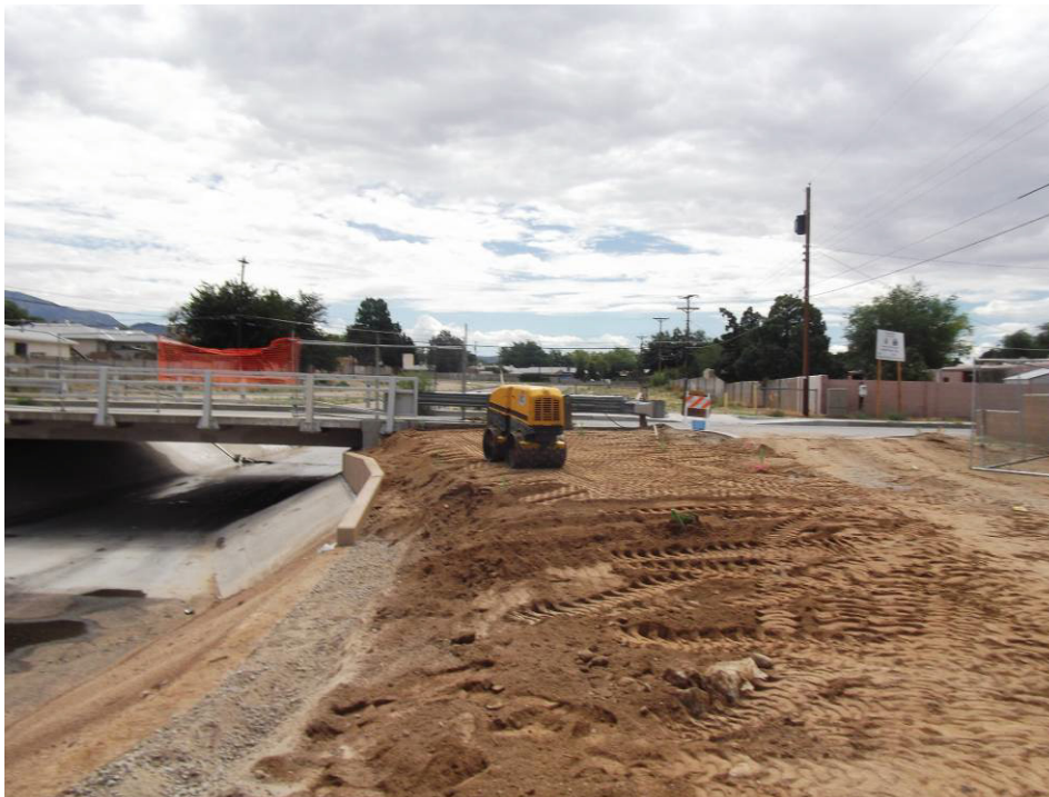
RMCI grading at California and backfilling against the sill wall on south side of the channel
