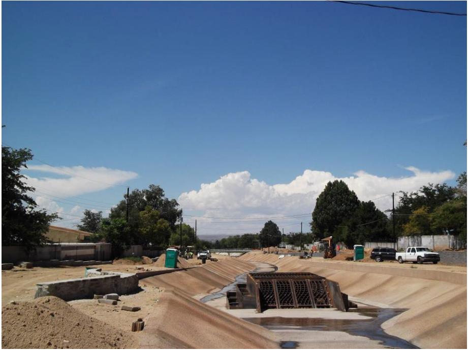
Leescapes finishing up the seatwall on the south side of the channel and Peerless working on "A" Wall on the north side
