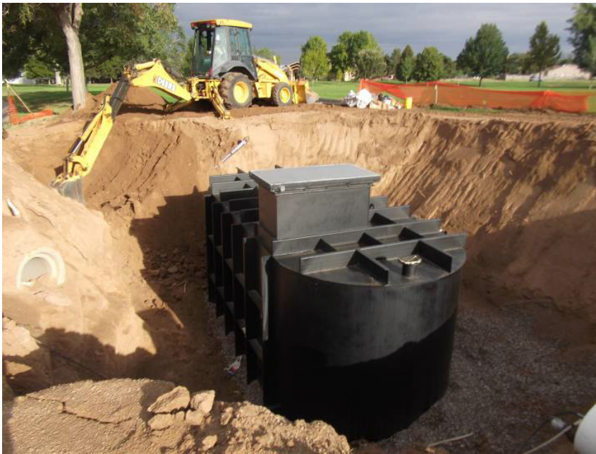
RMCI trenching to connect the 3" Di line that runs under the channel to WBS
