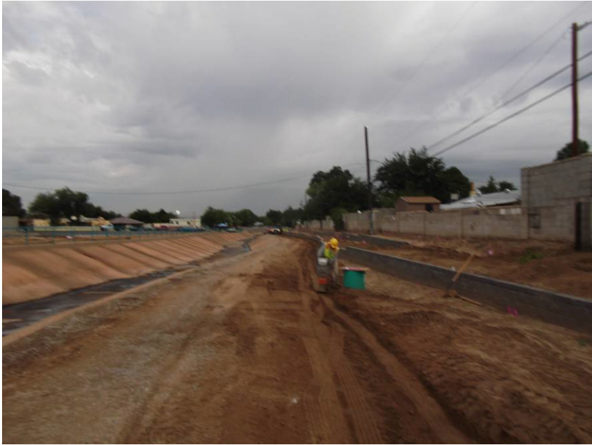
Land Tek backfilling the main irrigation line trench from San Pedro to California
