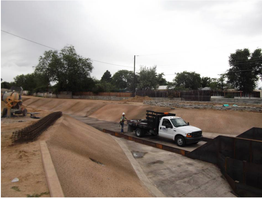
RMCI laying out and fabricating one foot low flow wings for welding tomorrow.
