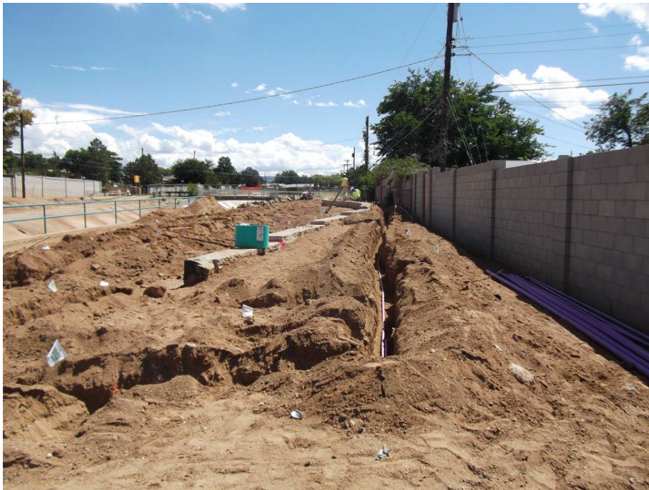
Land Tek placing lateral lines between California and the Church on the south side of the channel.
