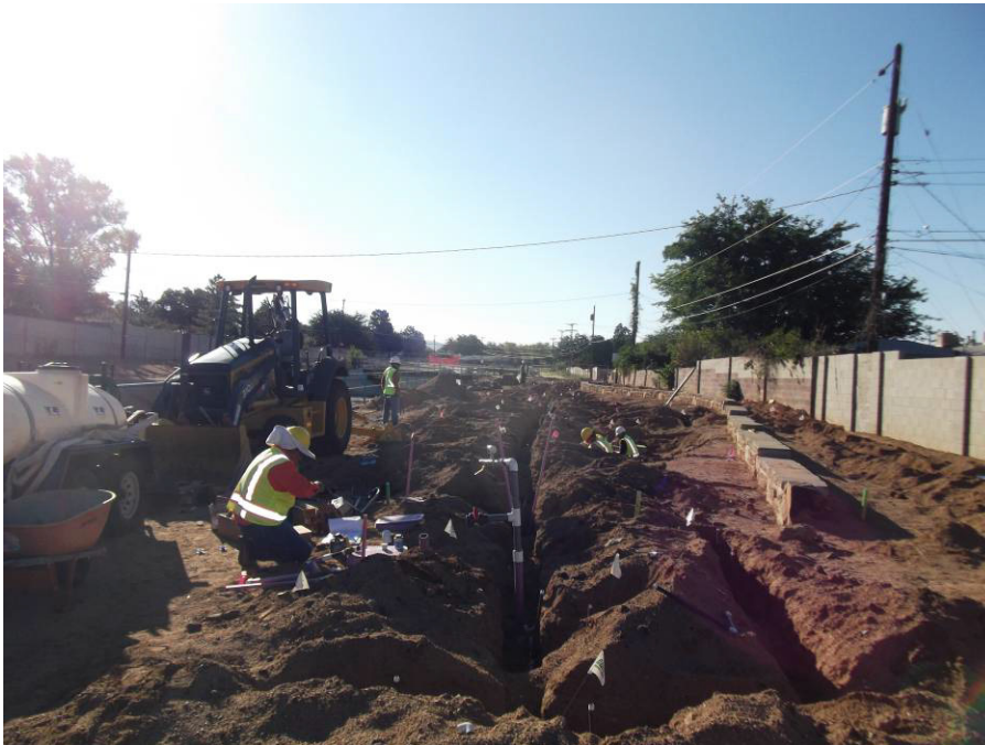
Land Tek trenching for lateral lines between California and the Church on the south side of the channel.
