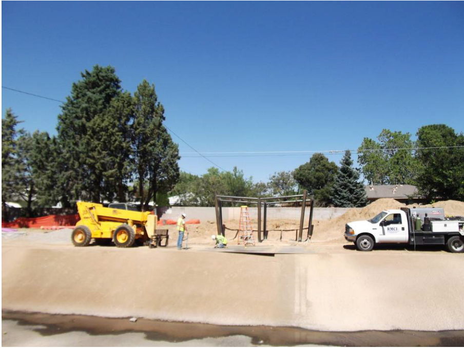
RMCI building the shade structure on the north side of the channel
