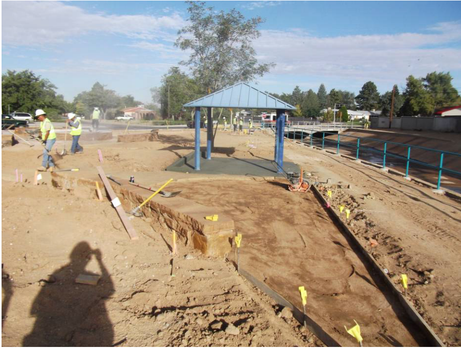
Bominate compacting area in the front of this photo. RMCI hand grading on the left side. Bominate saw cutting at the circular seat wall and HO laying out forms for exposed aggregate on the right hand side in the back of the photo.
