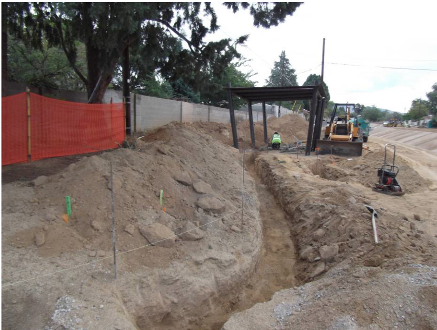
Leescapes placing base for the seat wall that runs under the shade structure.
