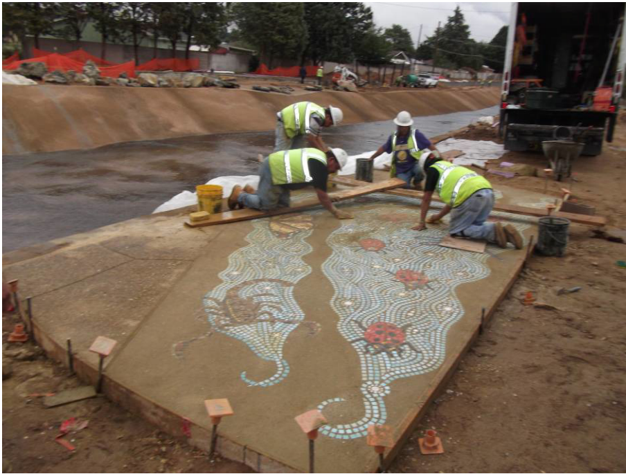
Bominate placing one of the art pieces in a plaza located on the south side of the channel just east of Comanche.
