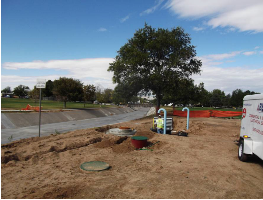
Bixby working with Bob, who is down in the booster station.
