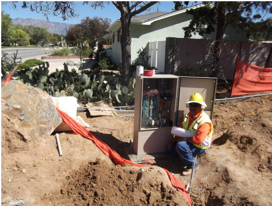
Land Tek working with Bixby to get power to the controller.
