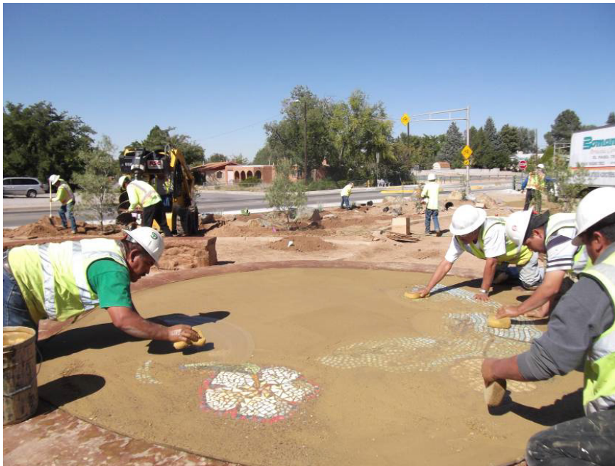
Bominite exposing the tiles on the seat wall in the pocket park.
