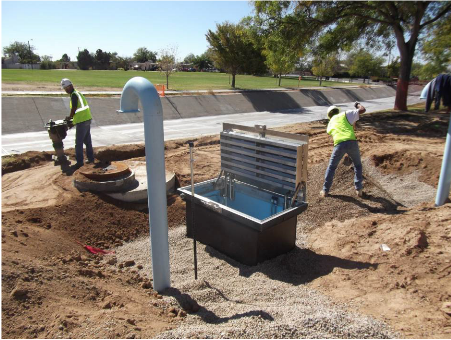
RMCI placing gravel around the manway of the water booster station. Antenna placed on the west side of the goose neck.
