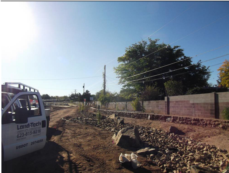
Land Tek placing rock in landscape areas on the south side of the channel west of California
