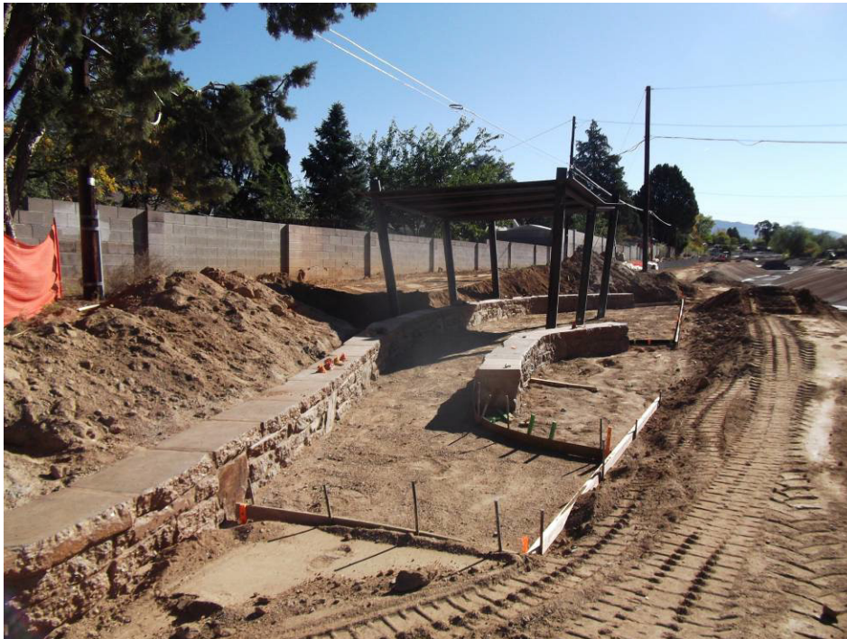
HO prepared subgrade and set forms for exposed aggregate under the shade structure.
