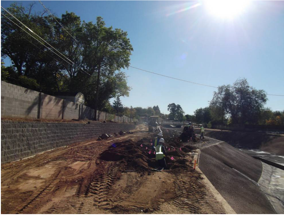
Land Tek trenching for laterals on the north side of the channel.
