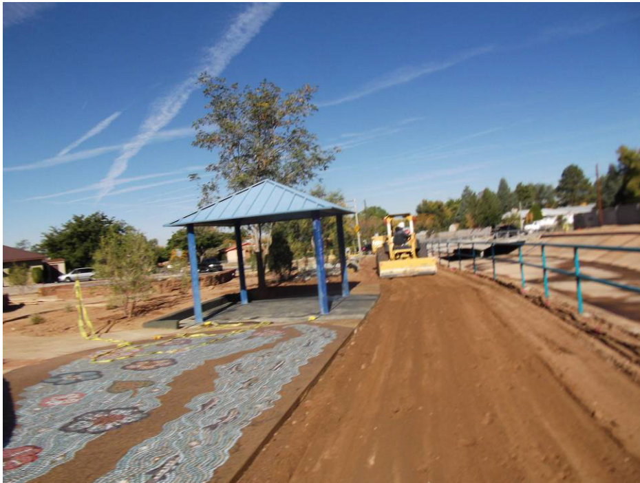
AAI preparing subgrade for the bike trail between San Pedro and California
