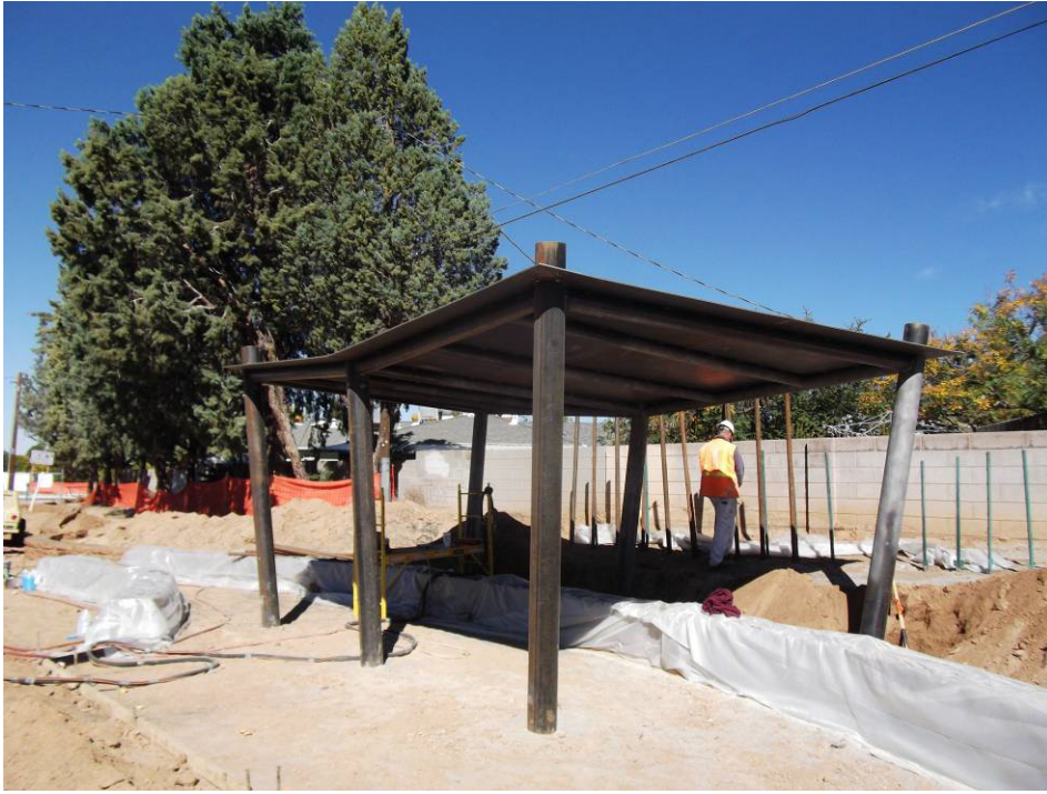
Gallery Paint sand blasting the shade structure. They covered the seat wall against damage.
