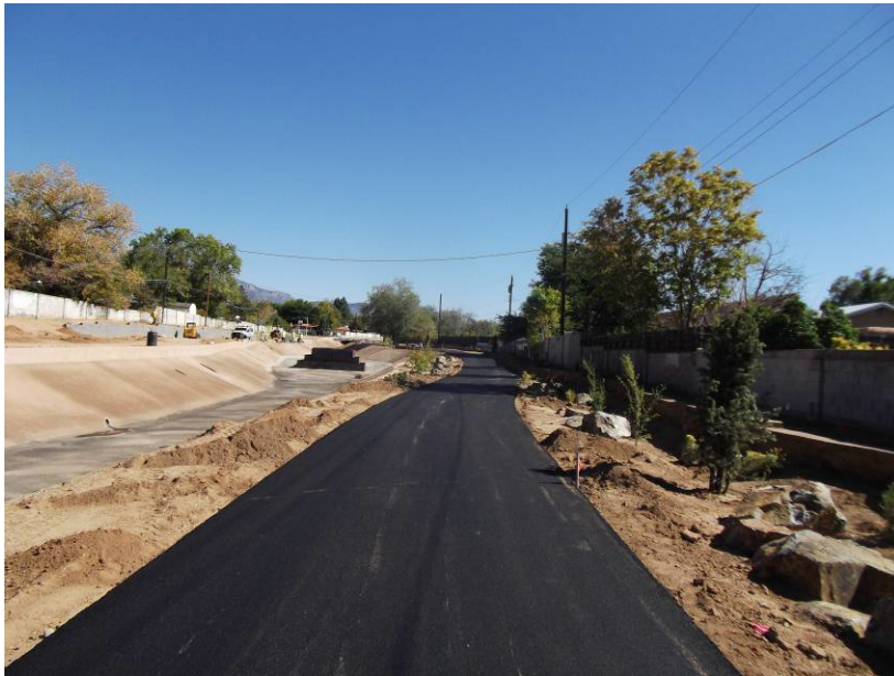
Paved bike trail on the south side of the channel between San Pedro and Comanche
