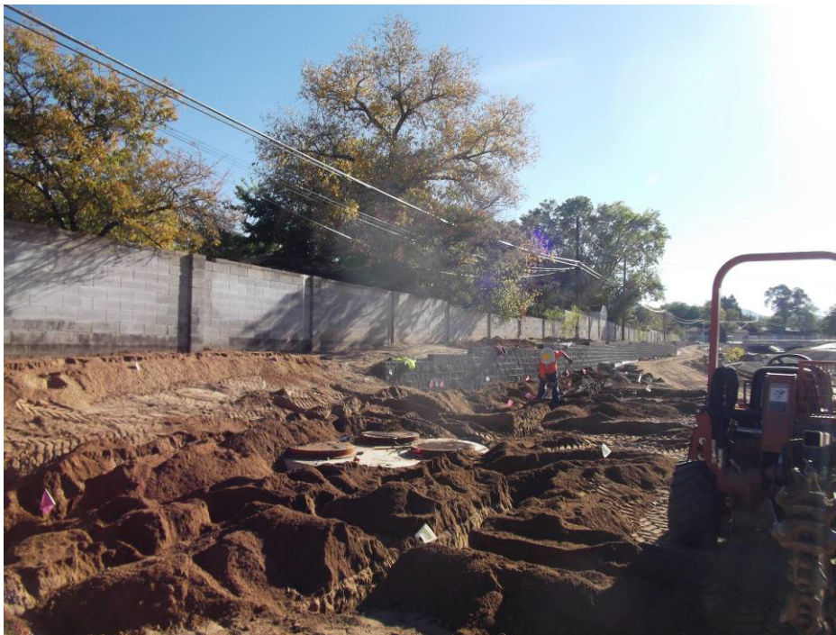
Land Tek trenching for laterals on the north side of the channel west of San Pedro.
