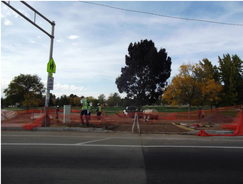
HO placing drive pad and sidewalk at Montgomery Park by the WBS
