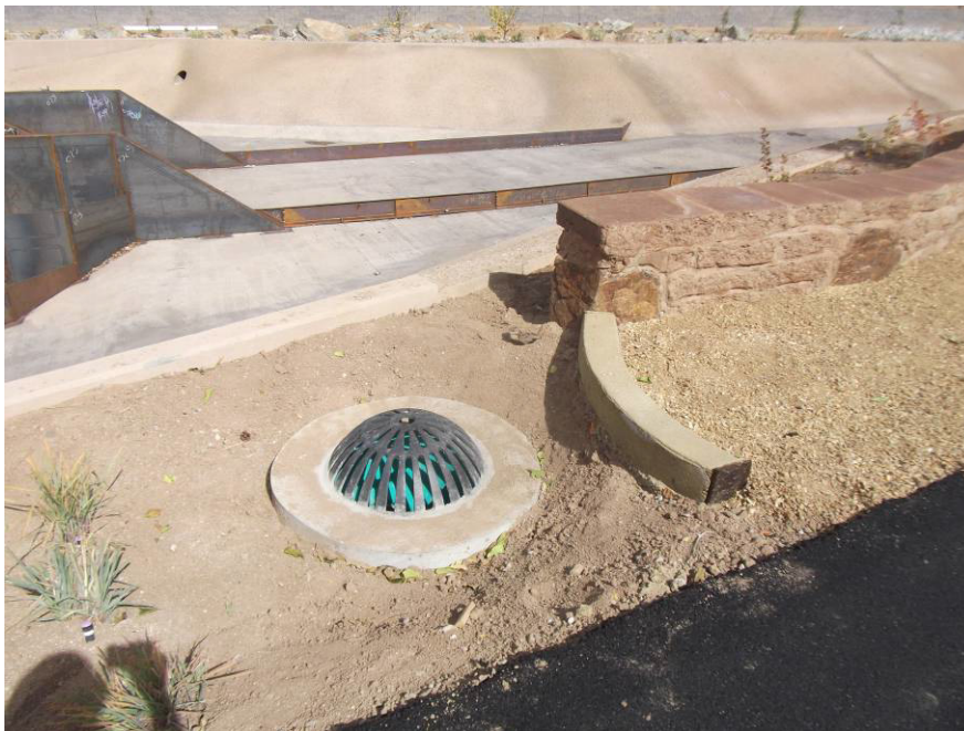
This area will need to be regraded for proper drainage.
