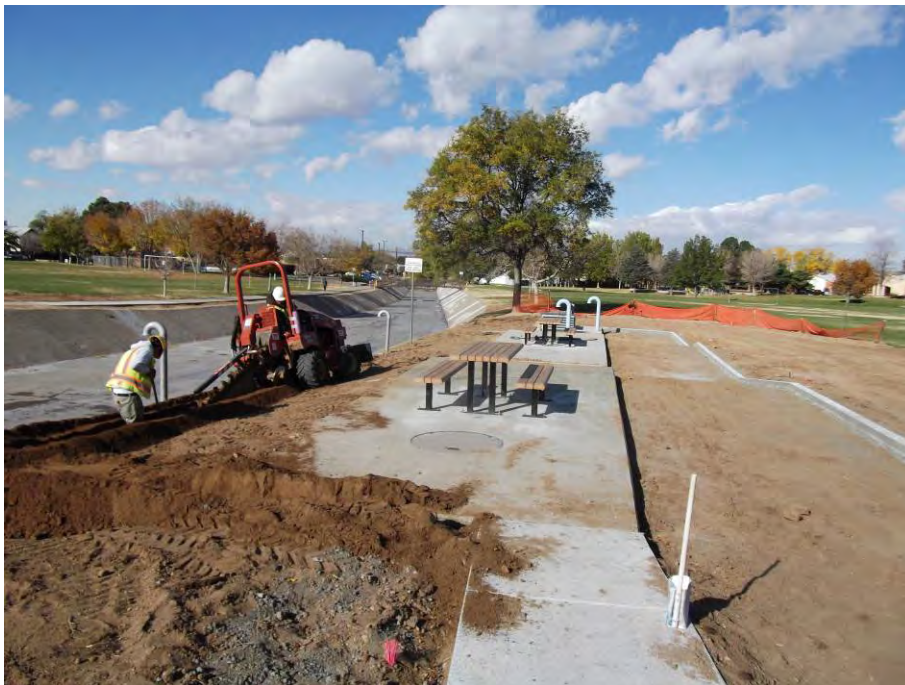
Land Tek trenching for new irrigation line. RMCI placed picnic tables over the weekend.
