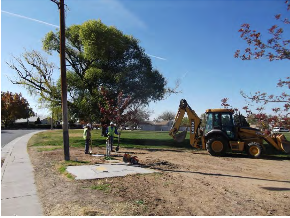
RMCI preparing to cut and cap the water line tie in at the south side of Montgomery Park.
