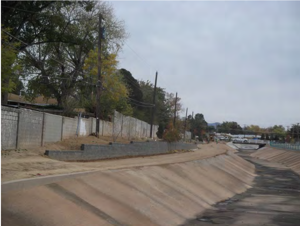
AAI finishing the dirt roadway on the north side of the channel.
