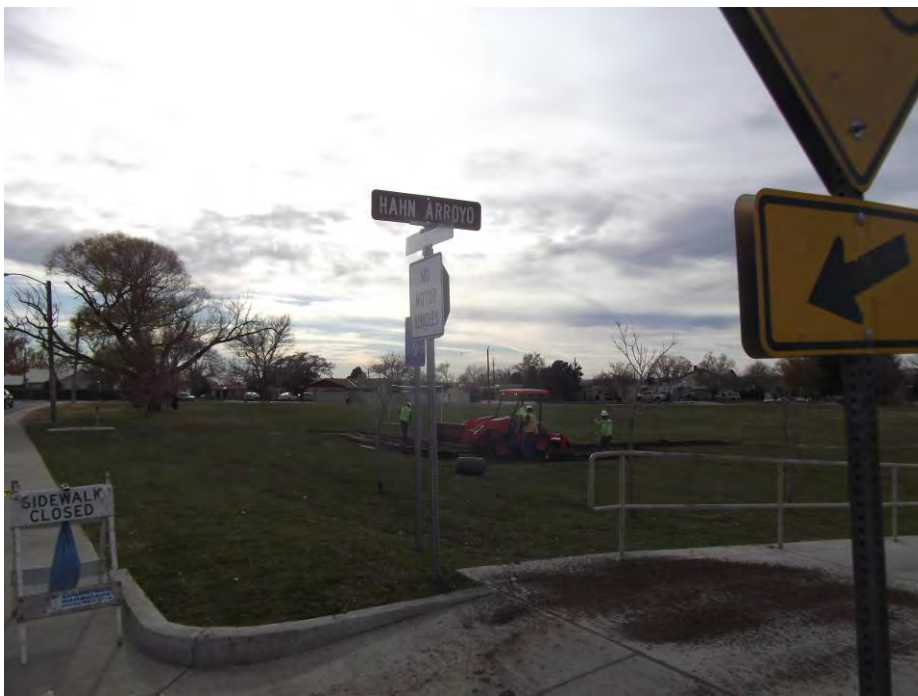
Land Tek placing sod on the south side of the channel at Montgomery Park.
