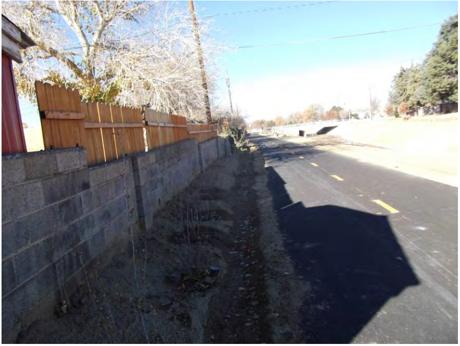
Drainage swale along the south side of the project located east of Comanche working well.
