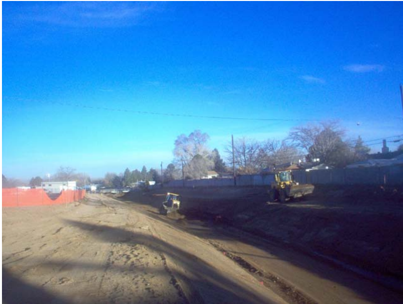
Guzman processing the bottom of the channel where waters saturated the subgrade.
