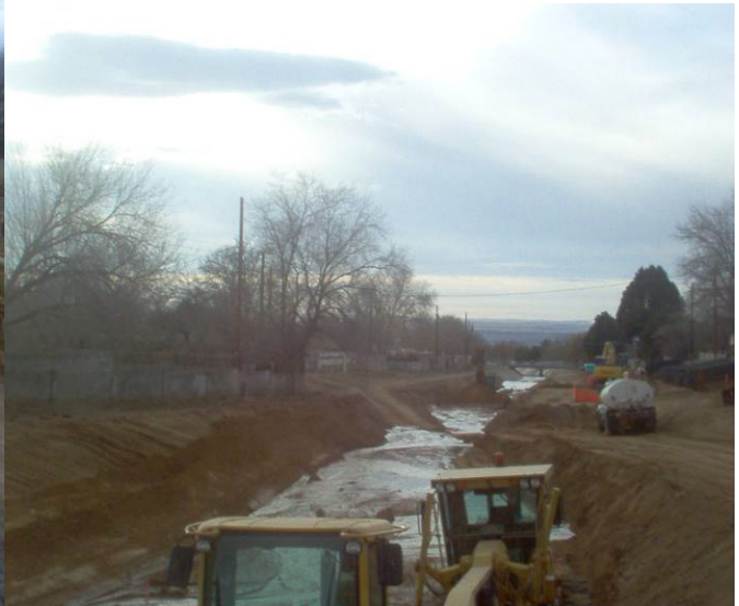
Waters are collecting around stockpiled debris and ramps.
