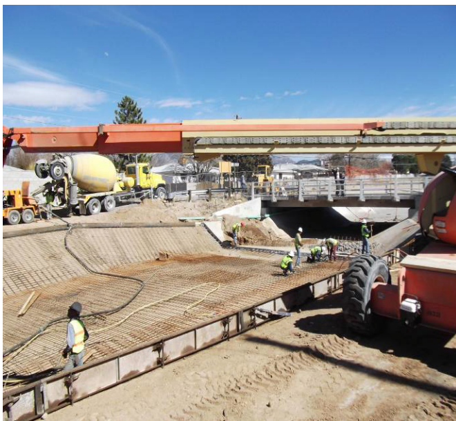
Tying rebar to existing, cleaning channel lining at tie in and shotcrete right behind.
