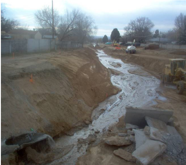
Waters running off of San Pedro due to fire hydrant being opened upstream on Colorado.
