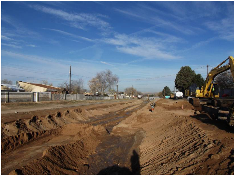
Guzman turning over the mud in the bottom of the channel. RMCI placing RCP on the right of the picture.
