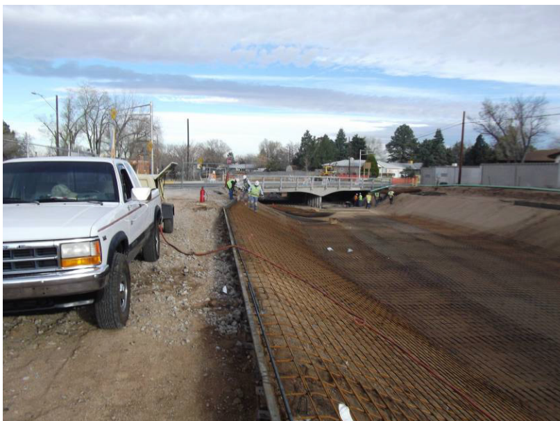
RMCI crews placing top forms, PRS placing rebar and Guzman removing channel lining under the bridge.
