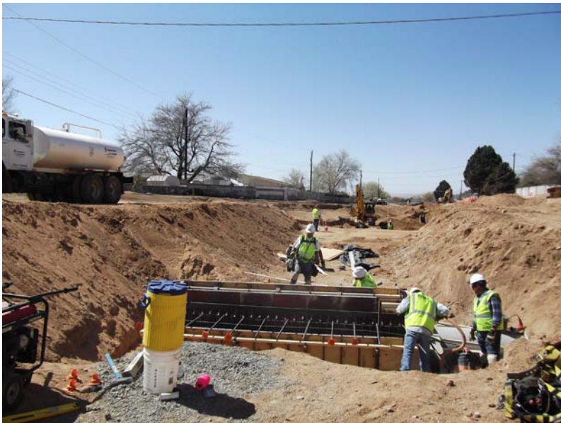
RMCI forming and preparing to pour the walls on the cattle guard.
