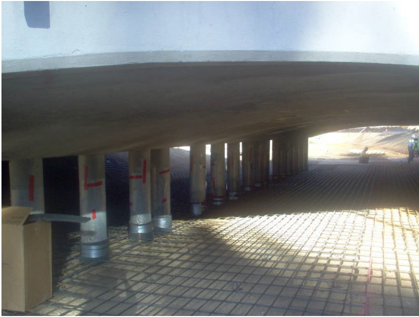
Under the San Pedro Bridge – Plastazote Expansion material placed and plastic hung to protect pilasters for easier clean up
