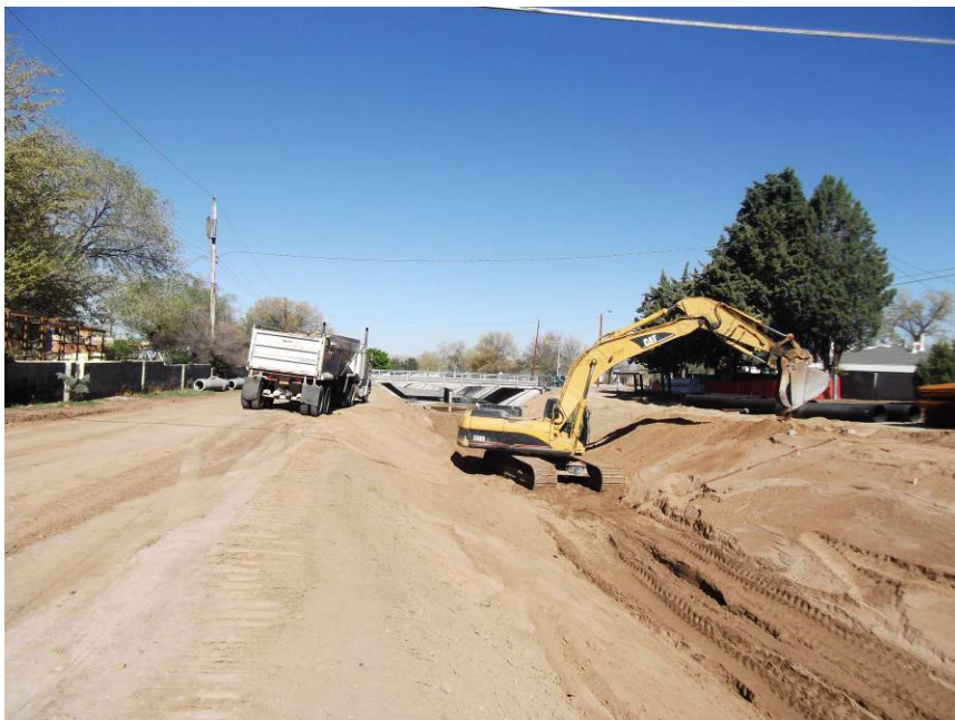
Guzman loading one truck of debris from the site. This should be the last of those removals.
